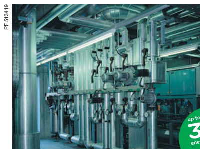
ATV12 controlling a pumping station
