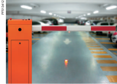
ATV12 controlling an access barrier
